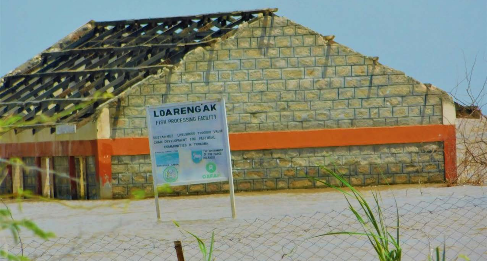
Lowarengak Beach Management Unit offices in the northern sector of Lake Turkana destroyed by strong winds and increased lake levels. Photo by James Last.
