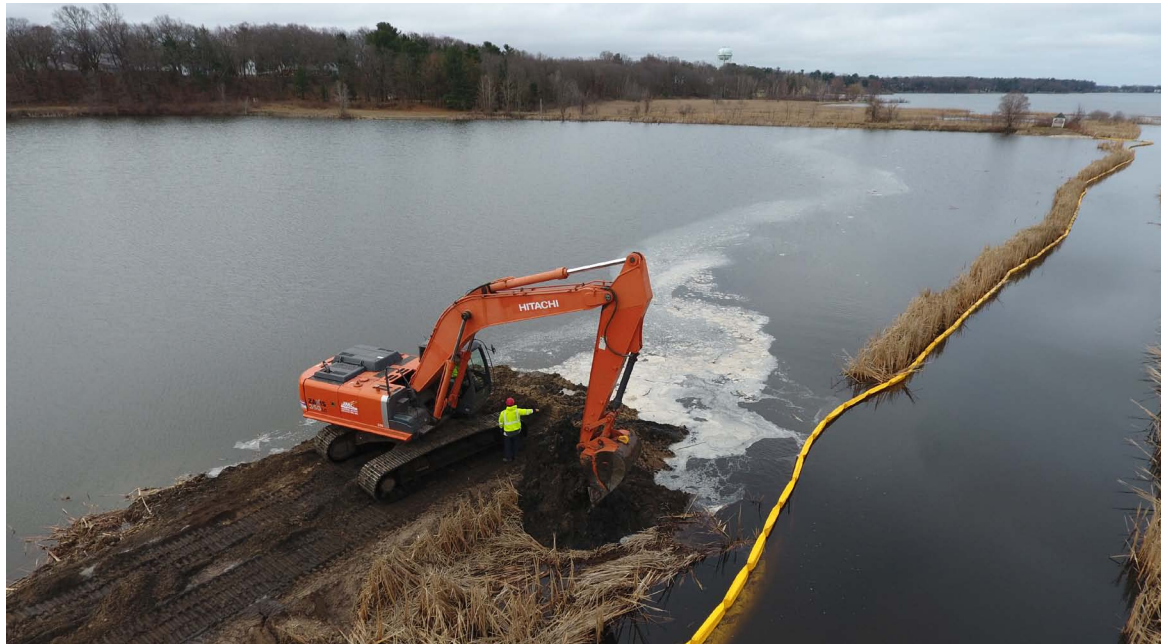
Berm removal to restore hydrological connection to Bear Lake. Credit: GEI Consultants of Michigan.
